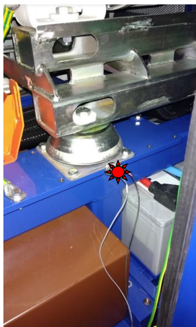
Fig. 9.7. B2 Measurement point B level 2 under the insulator, generator side
