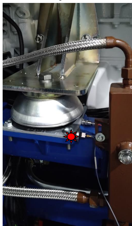
Fig. 9.3. A2 Measurement point A level 2 under the insulator, engine side
