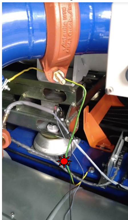
Fig. 9.15. D2 Measurement point D level 2 under the insulator, generator side
