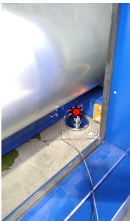
Fig. 9.12. C3 Measurement point C level 3 measurement base of the unit frame
