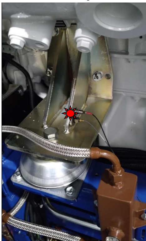
Fig. 9.2. A1 Measurement point A level 1 above the insulator, engine side
